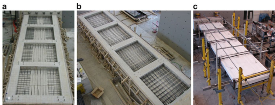
Fig. 16.2 Specimen no. 1: (a) frame with long starter bars and short dowels per option (a) along the top and one lateral side of each panel and the long dowels per option (b) along the other two; (b) two-way reinforcement placed in the new web; (c) specimen in testing position with actuators and sensors attached
