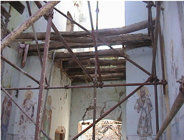
Fig. 8.14 Damage to the floor structure
