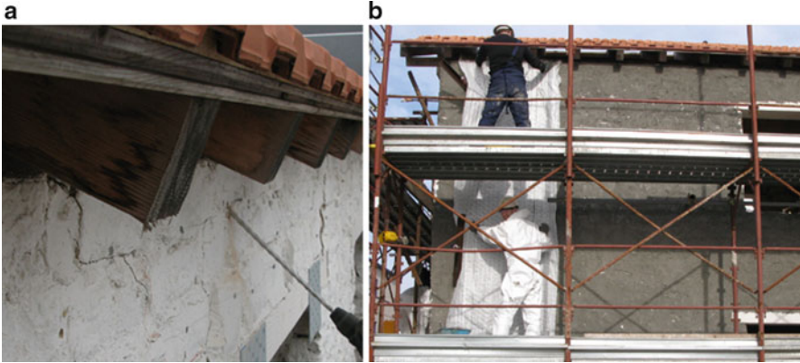
Fig. 9.11 (a) Borehole drilling for steel anchor connection between masonry and roof; (b) application of textile layers in vertical orientation
