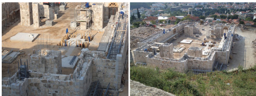
Fig. 8.27 Construction of the church up to the level of first horizontal ties
