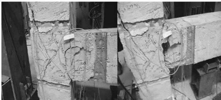
Fig. 13.15 Formation of crack in joint during cyclic load test of specimen J-BI-18
